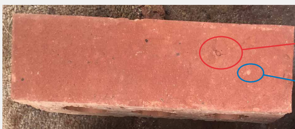
Figure 2 – The same brick with a remedial tint application and natural weathering.
